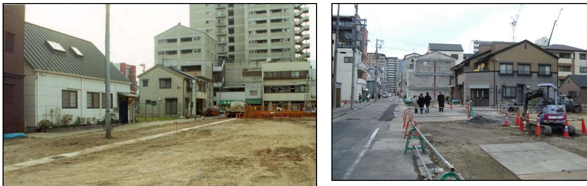
Figure 7-34: (a) Street widening (from 2 to 6 meters) in progress in June 2000 (note utility pole's location in the middle of new street); (b) Street widening underway in January 2003 (note offset buildings)
