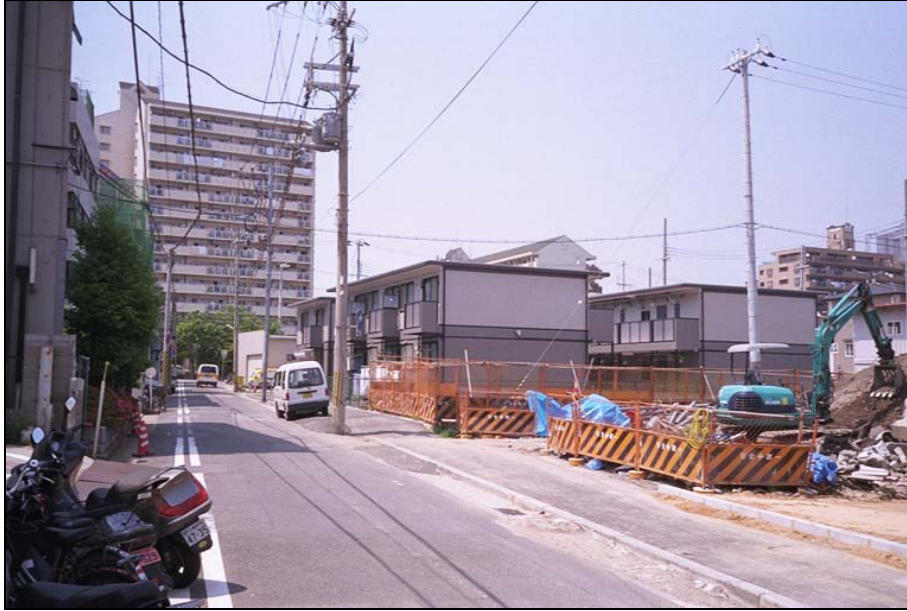
Figure 8-13: Kobe City post-earthquake public housing project in the background. Temporary housing and land readjustment in progress in Misuga West, June 2000
