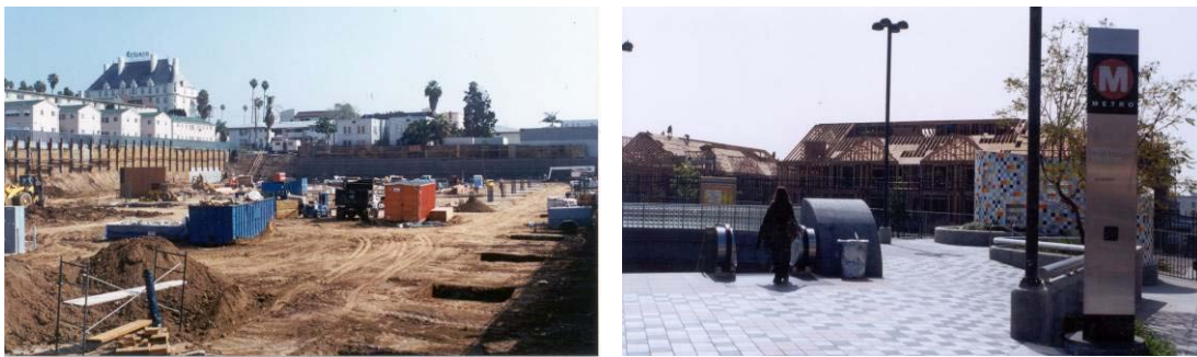
Figure 4-19: Hollywood and Western projects underway in March 2000 on (a) southeast corner and (b) northeast corner
